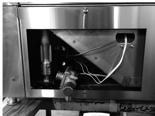
Rear Access Panel Removed
