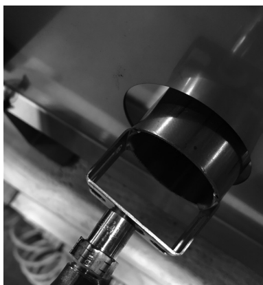
HEARTH BURNER NOT PROPERLY SEATED
