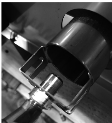
HEARTH BURNER PROPERLY SEATED
